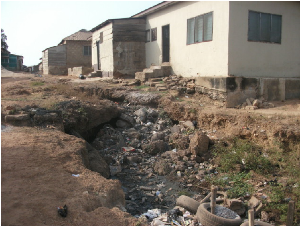
Figure 6: Buildings at risk due to gully erosion (source: author's fieldwork, December 2012)
