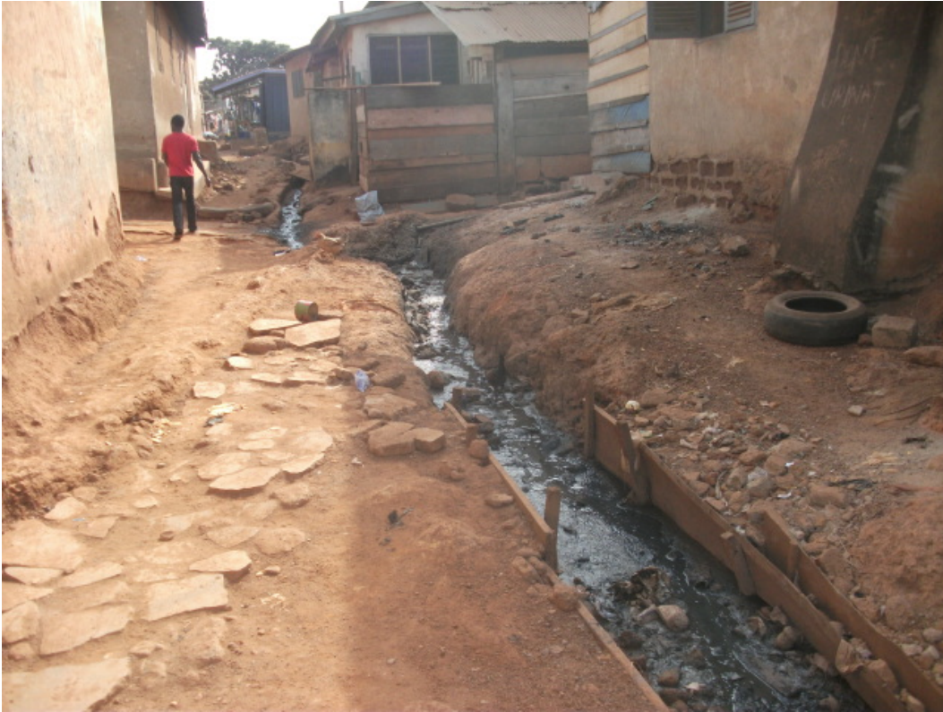
Figure 5: Poor drainage system in a section of Sunyani Area 2. (Source: author's fieldwork, December 2012)
