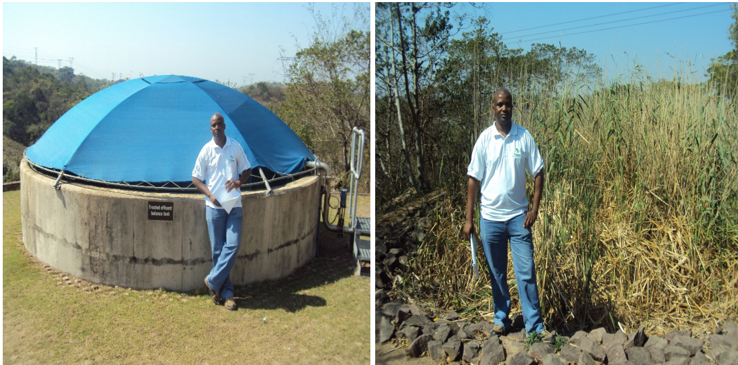
Figure 3: Leachate treatment plant and the reed bed that purifies waste water from the landfill site
